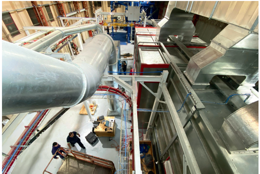
The plant in Córdoba, Argentina, was set up in close cooperation with Mankiewicz and WIWA. The new paint line was built by the company Göttert.
